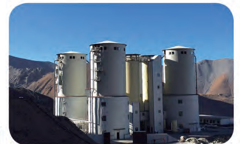
立式砂仓高浓度膏体充填料浆制备系统 Vertical sand silo high-concentration paste backfill slurry preparation system
